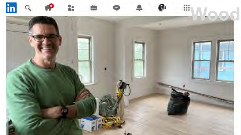
DCVL Design Principal/CFO David Tomás De Celis on site of a current renovation project in Cambridge, MA. © D.T. De Celis
