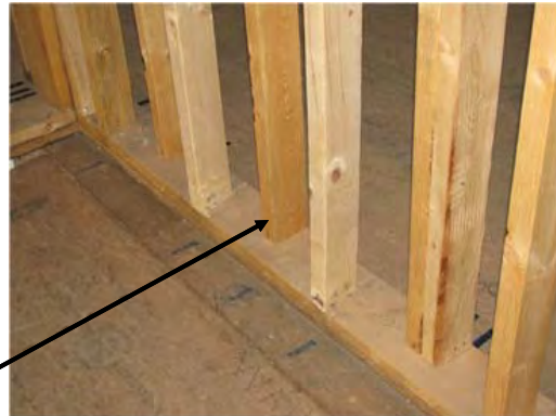
GAP ALLOWS SMOKE AN FIRE SPREAD BETWEEN CAVITIES
